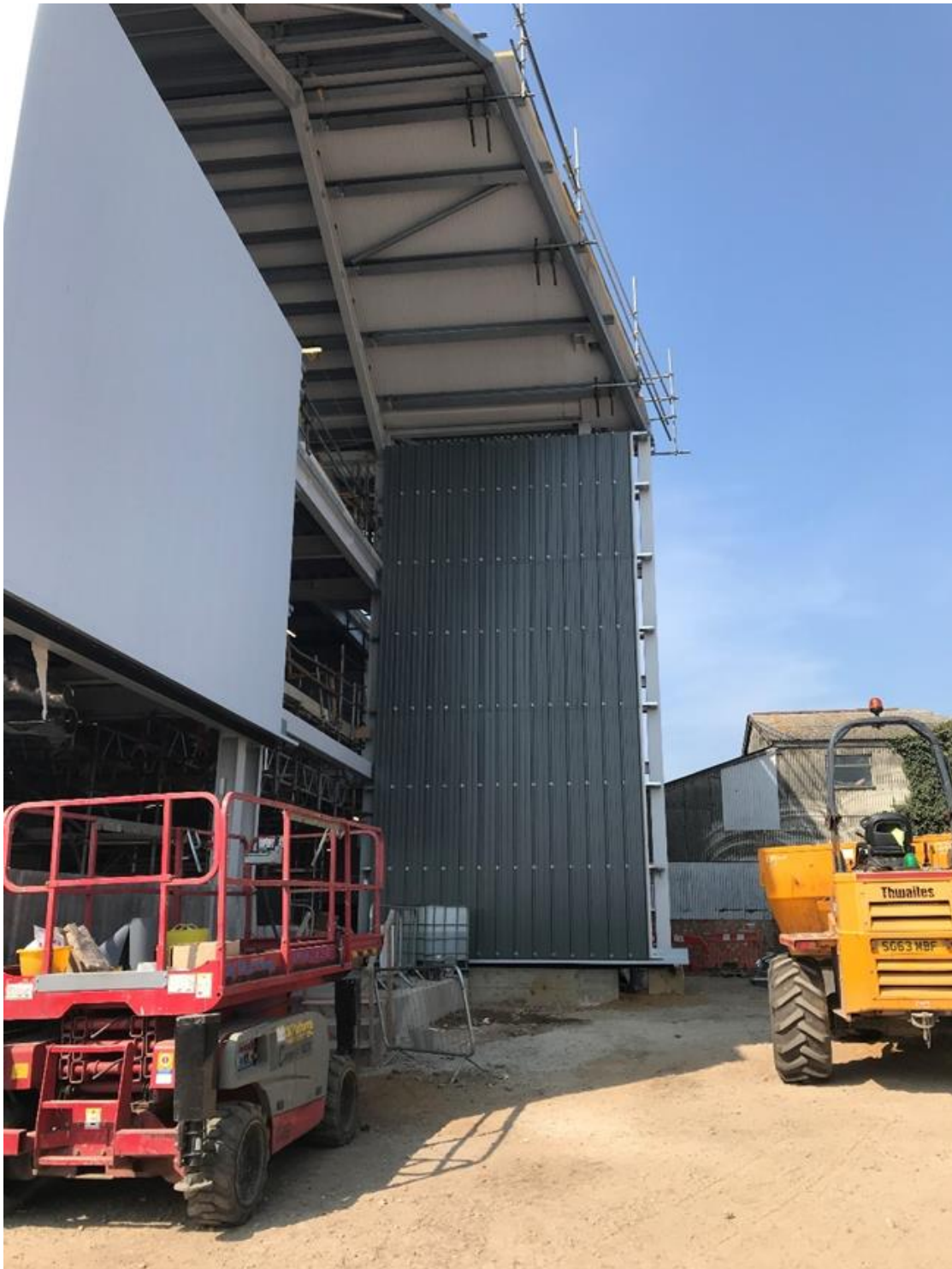
Plate 6.2 Example of dark grey composite cladding used on a substation office building (example taken from construction of East Anglia ONE substation)
